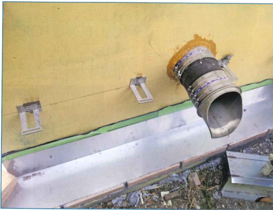
Photo 8 - Fluid-applied WRB and flashing at pipe penetration and brick ties in process. Photo courtesy of STO Corp.
