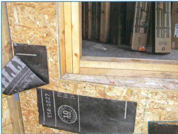
Photo 11 – A fluid-applied flashing application to recessed window opening. Step 1: Fasten sheet WRB.
