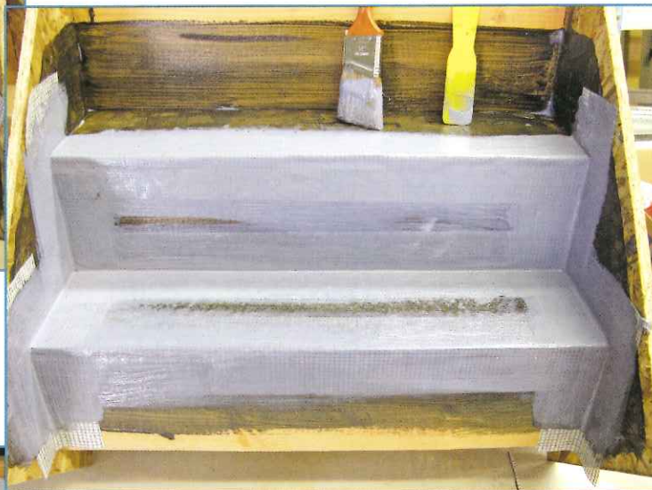
Photo 17 – Lay fabric into a coat of acrylic, typically working from bottom up. Smooth with overcoat.
