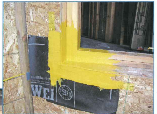
Photo 13 – Recessed window flashing. Step 3: Apply liquid flashing to opening and spread smooth.
